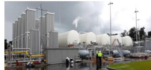
LNG reloading and bunkering station in Klaipeda
